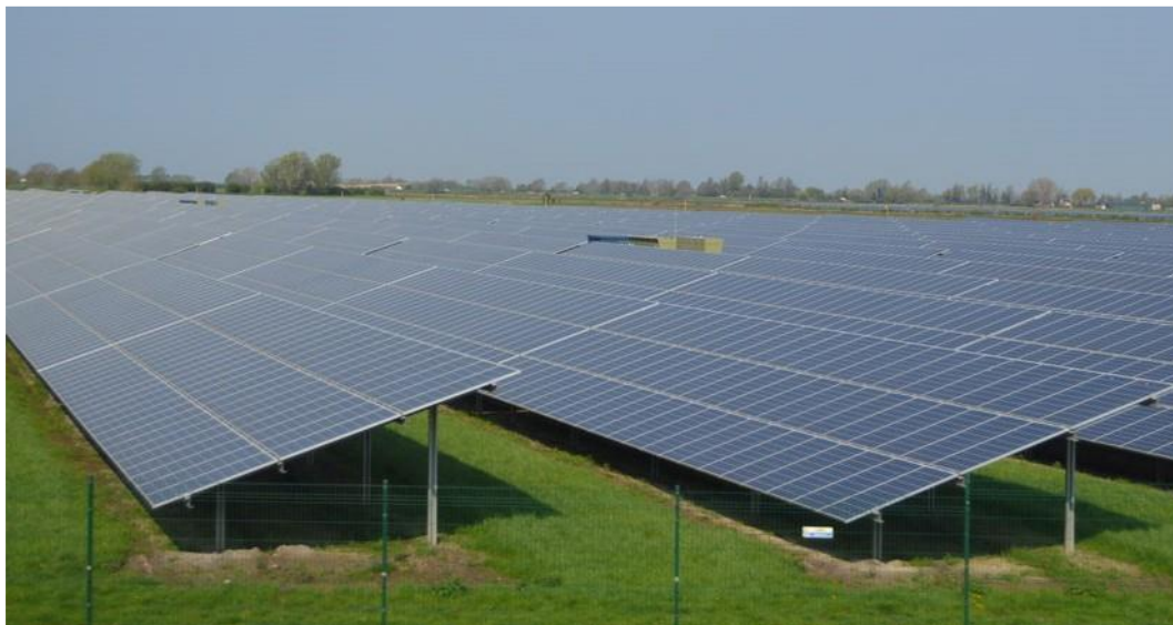
Image 3.1 – Example Solar PV Panel Arrangement
