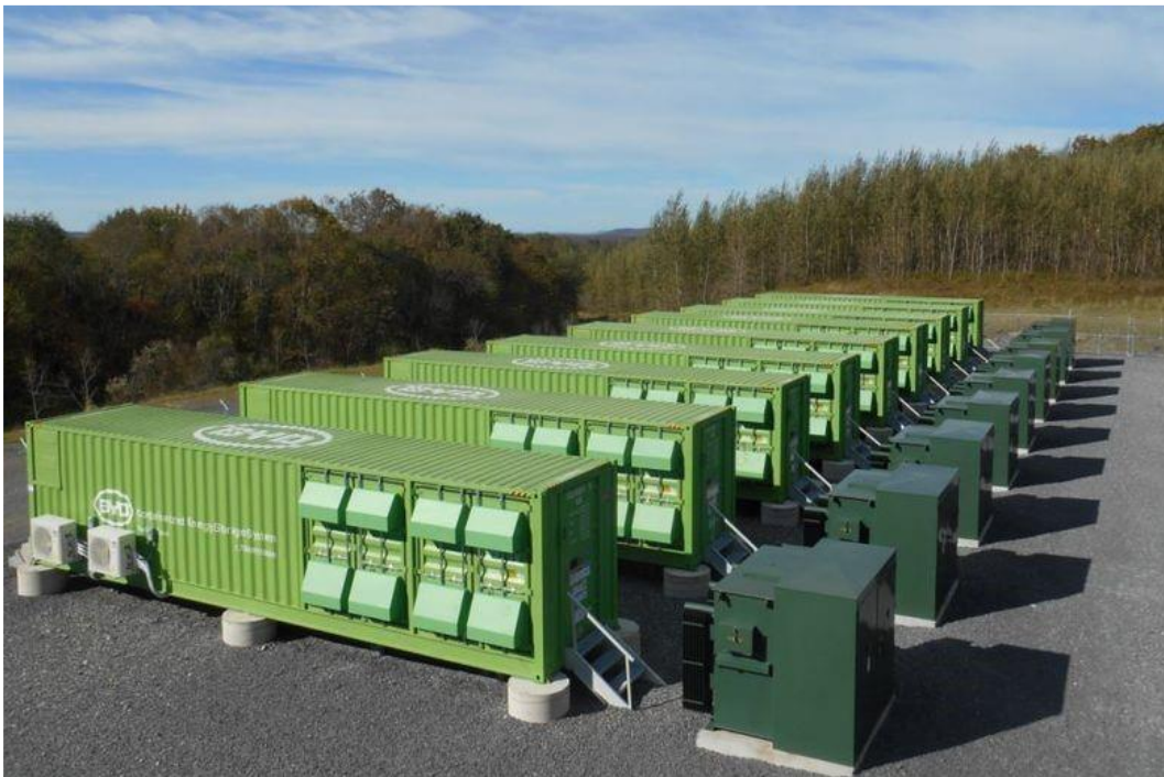
Image 3.4 – Example BESS Facility
